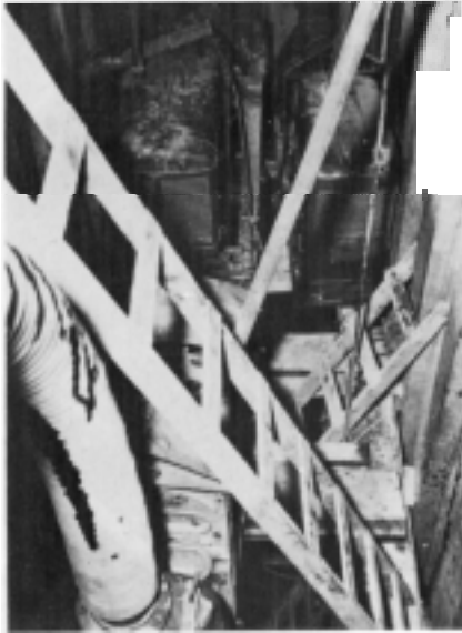
Figure 73. The 4,100-gallon-per-minute pump used to dewater cofferdam 4 so that the lower whaler could be installed.
