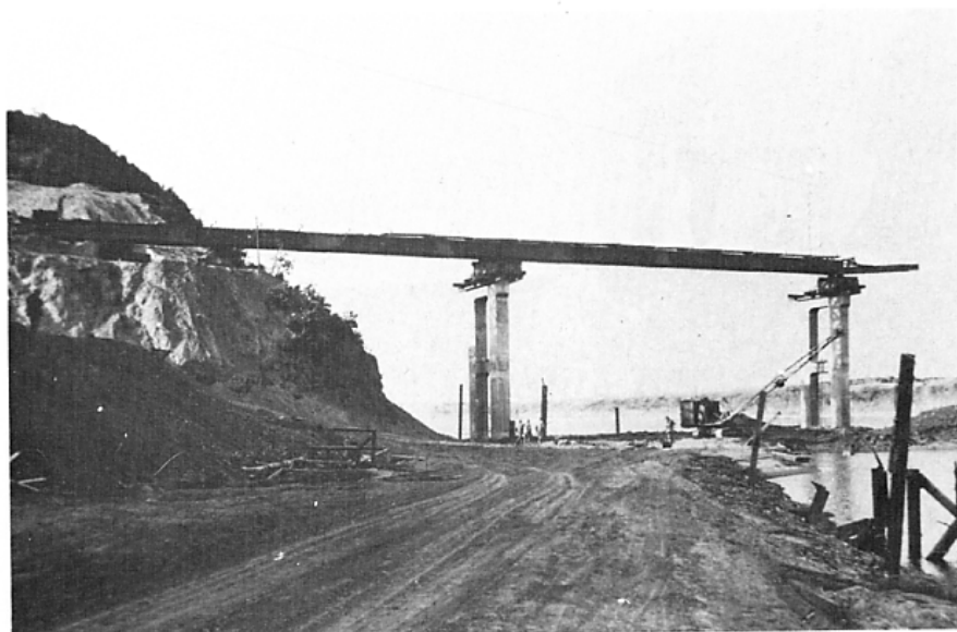
Figure 53. Steel beams in place from the west abutment across pier 8 to pier 7. The 30-foot launching nose may be seen beyond pier 7.
