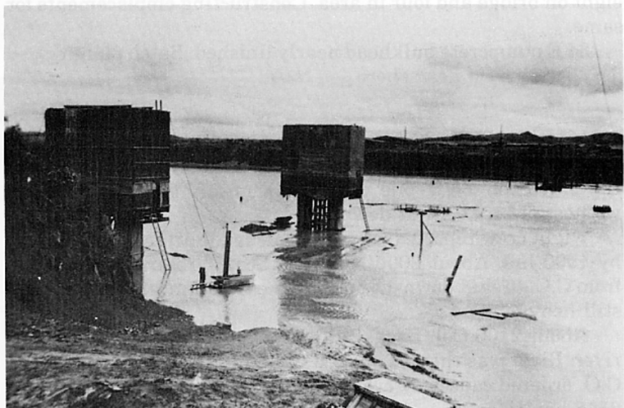
Figure 67. Storm water and a spring high tide combined to force an evacuation of the causeway on 20 March 1953. Piers 7 and 8 are in the foreground.
