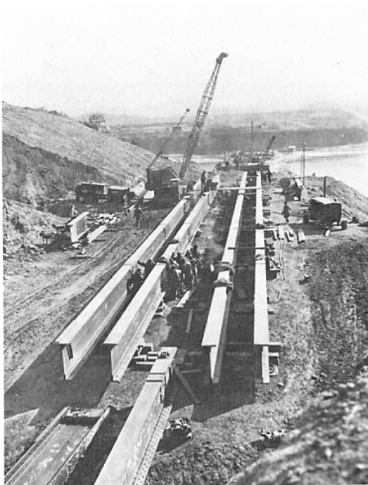
Figure 52. Steel beams being prepared for the span from the west abutment to pier 7, while riveters received training on the beam at left center.
