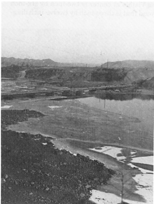
Figure 31. Teal bridge from the south shore on 7 January 1953 as troops place decking on the north end.
