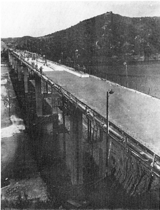
Figure 59. Concrete deck being covered with burlap, at center, prior to receiving a seven-day water cure. A flood gauge is visible on pier 1 in foreground.
