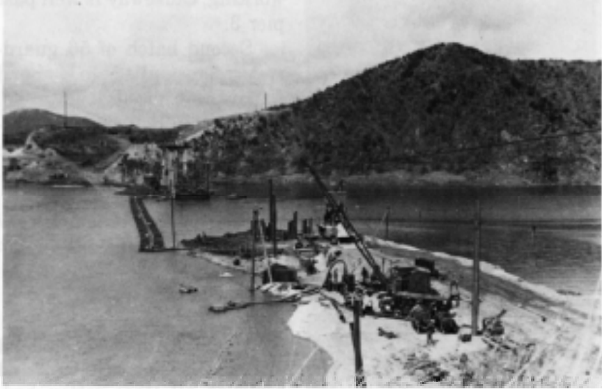
Figure 70. View of the footbridge that enabled the pumpcrete machine to pump concrete from its location near pier 3, at center, to pier 6 across the river channel.
