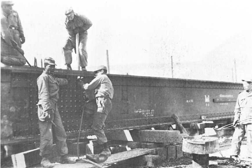
Figure 51. Riveters at work on steel beams. Newly trained American and Korean riveters developed their skills so quickly that a 121-foot span was launched with a deflection of only 17 inches.
